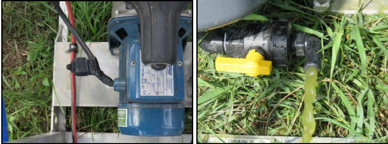
Figure 37. First Response Pump Motor Circuit Breaker (left) Backwash Output (right)
